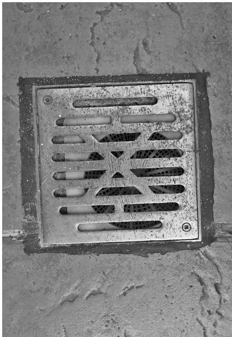
FIGURE 2.14 A standard grate. Note the smaller plastic mesh placed underneath, as recommended by local authorities, to prevent the passage of scorpions. (Photo by author)
